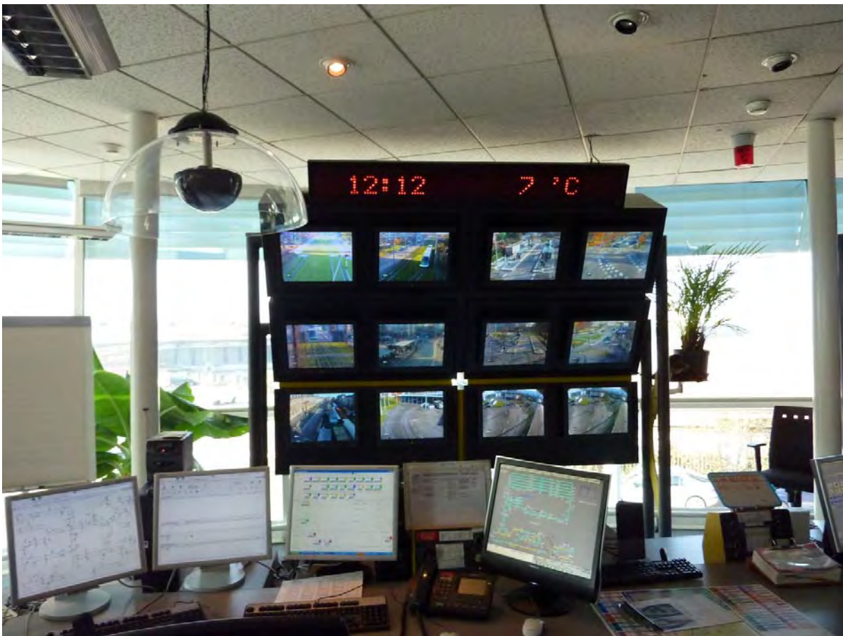
Figure 9 : Photo PCC Tramway Strasbourg
