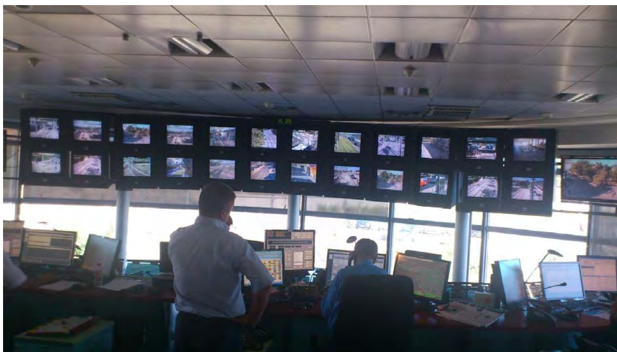
Figure 8 : Photo PCC Tramway Montpellier
